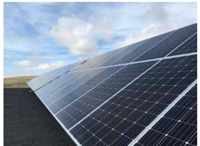
Some of the newly installed solar panels at KEC's Community Solar Project.
